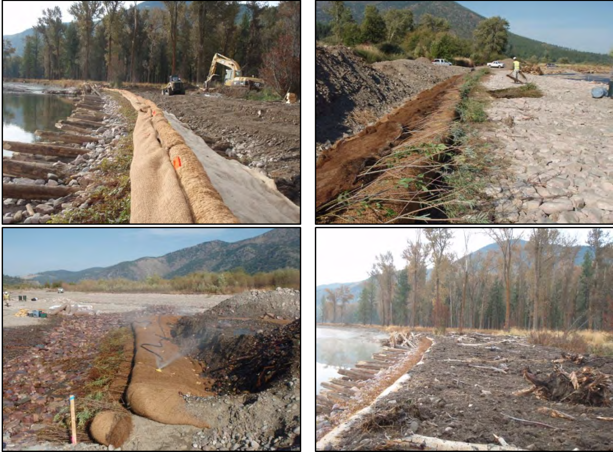
Figure 10. Photo series from left to right and top to bottom showing the construction of a vegetated soil lift.
