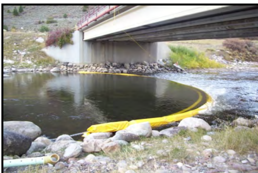
Stationary floating silt curtain installed at the downstream end of the project.
