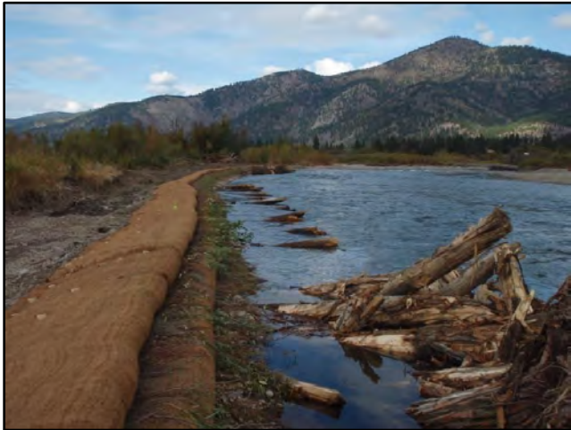
Figure 11. Photo showing a completed vegetated soil lift with a woody debris jam in the foreground and a log toe.
