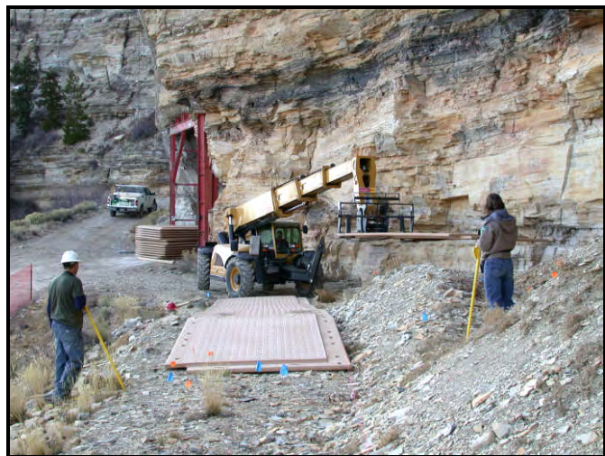
Figure 2. Positioning Dura-Base ® synthetic mats to create a driving surface and protect 33 penstemon.
