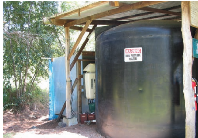
Figure 10.6 —Black water storage tanks are a low-cost way to warm irrigation water with solar energy before it is applied to crops. Photo by Thomas D. Landis.
